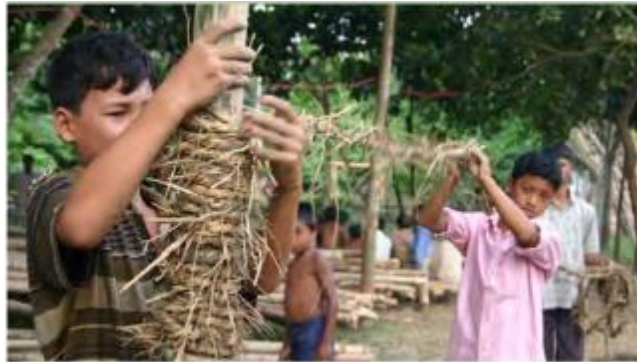
Figure 5-84 METI School Kids are learning to build, helping on site and so becoming a living part of the building (Lim, 2007).
