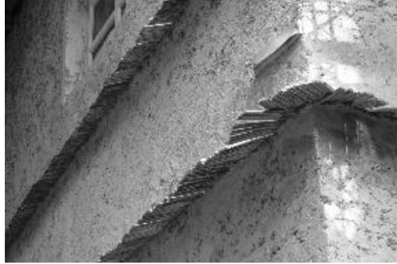
Figure 5-80 Bamboo and straw are used to slow down the erosion of the earth walls (World, 2015)
