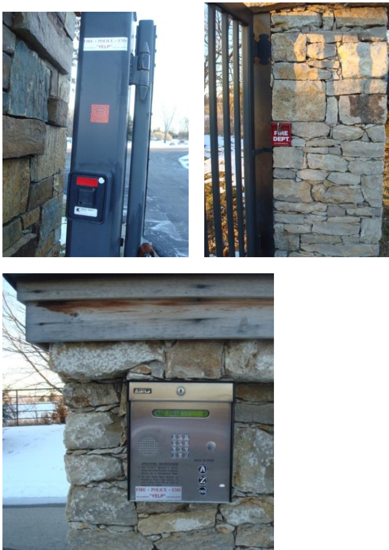
Figure 5-1 Knox Box, Fire Department Lock, Key Pad with YELP Sign
