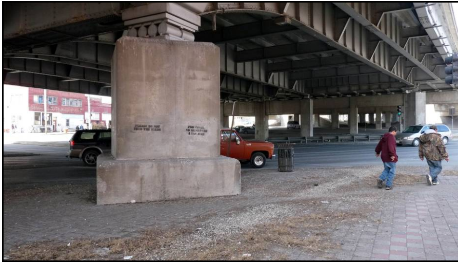
Figure 2.12. Conditions created by pigeons under I-35 overpass.
