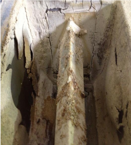
Figure 1.5 Feeder with potential contamination
