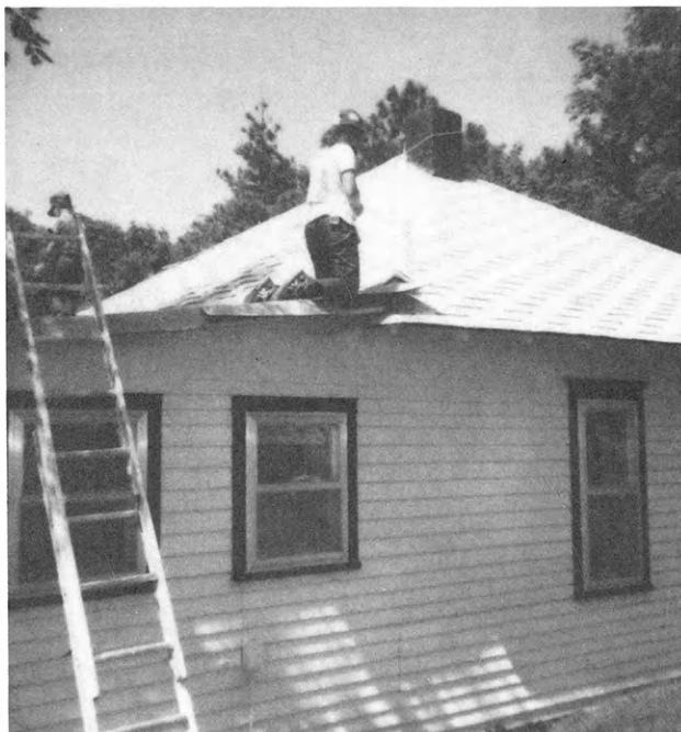
Janay Dunham nears the end of the roofing job she and her family did themselves. Notice the rope around Janay's waist which is attached to the chimney.
