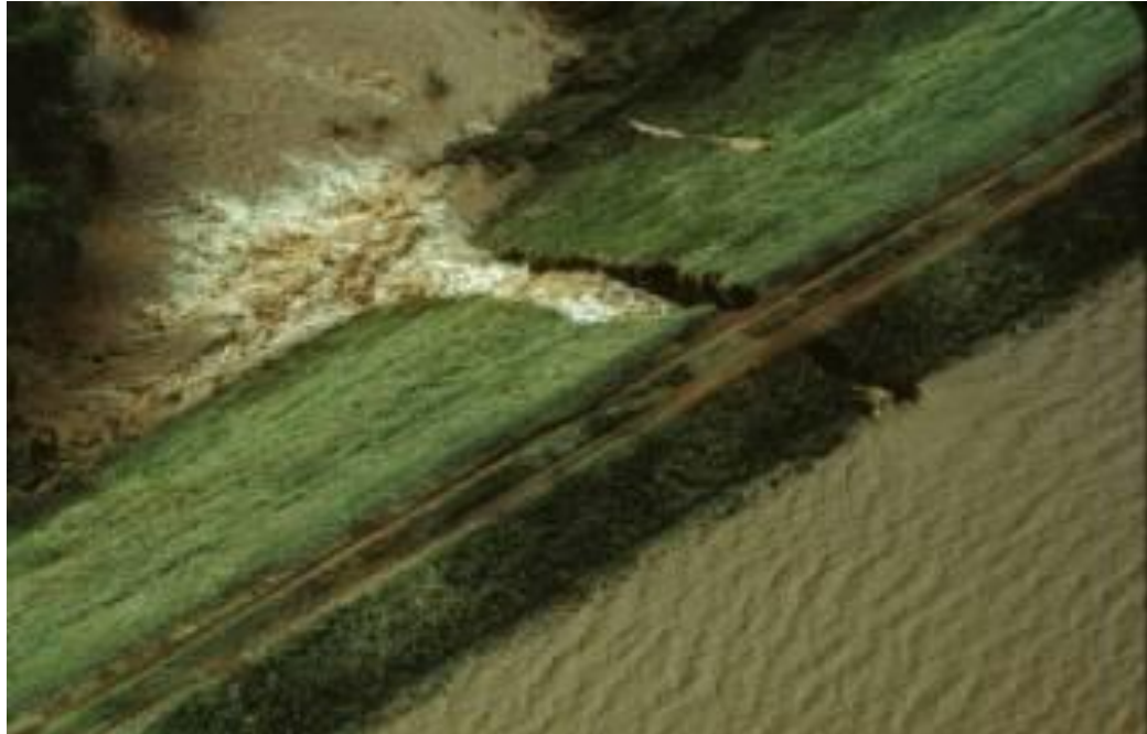
Figure 3. Internal Erosion of USDA NRCS Structure
