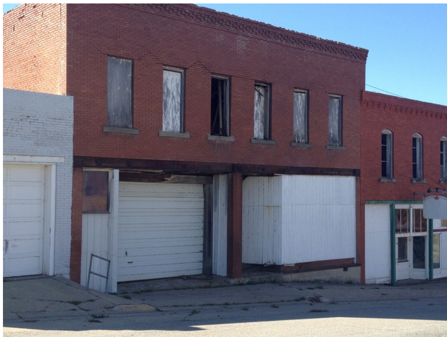
This is a photograph illustrating quality of sidewalks along Main Street. Figure 7. Current condition of sidewalk infrastructure (Photo by Author, 2012).
