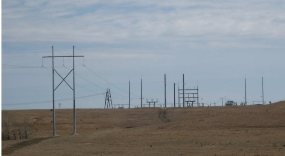
Figure 6.1: Power Lines at Meridian Way Wind Farm, Concordia, Kansas
