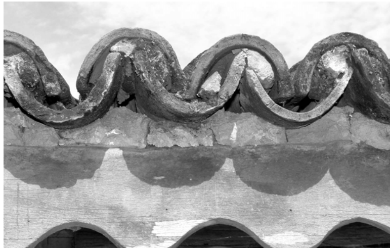
Figure 10. Author's photograph showing intercepting traditional roof tiles, khapada , with mud in-between, July, 2010.
