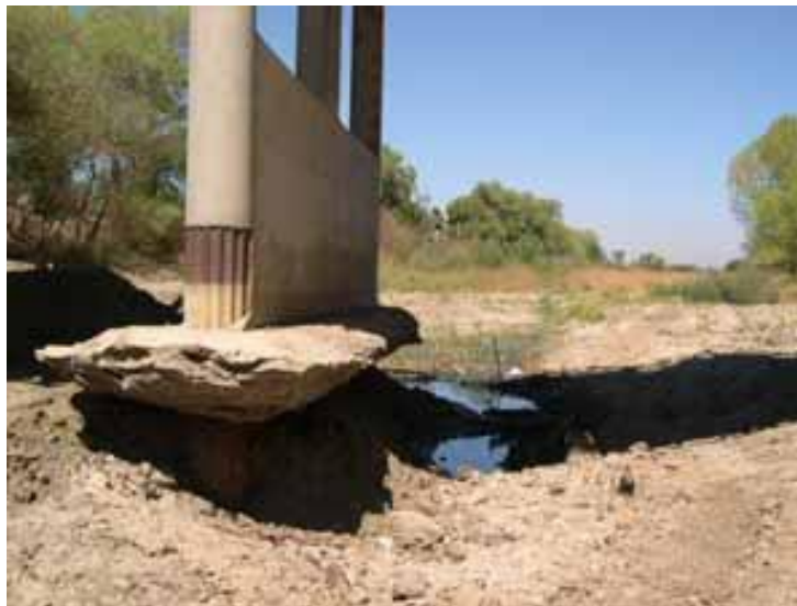
Fig. 1 Scour developed around bridge pier (Johnson 2015)
