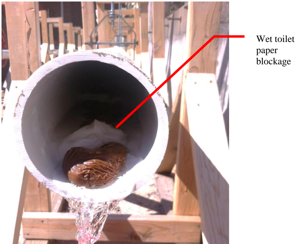
Figure 3.5 Pipe Clog Example
