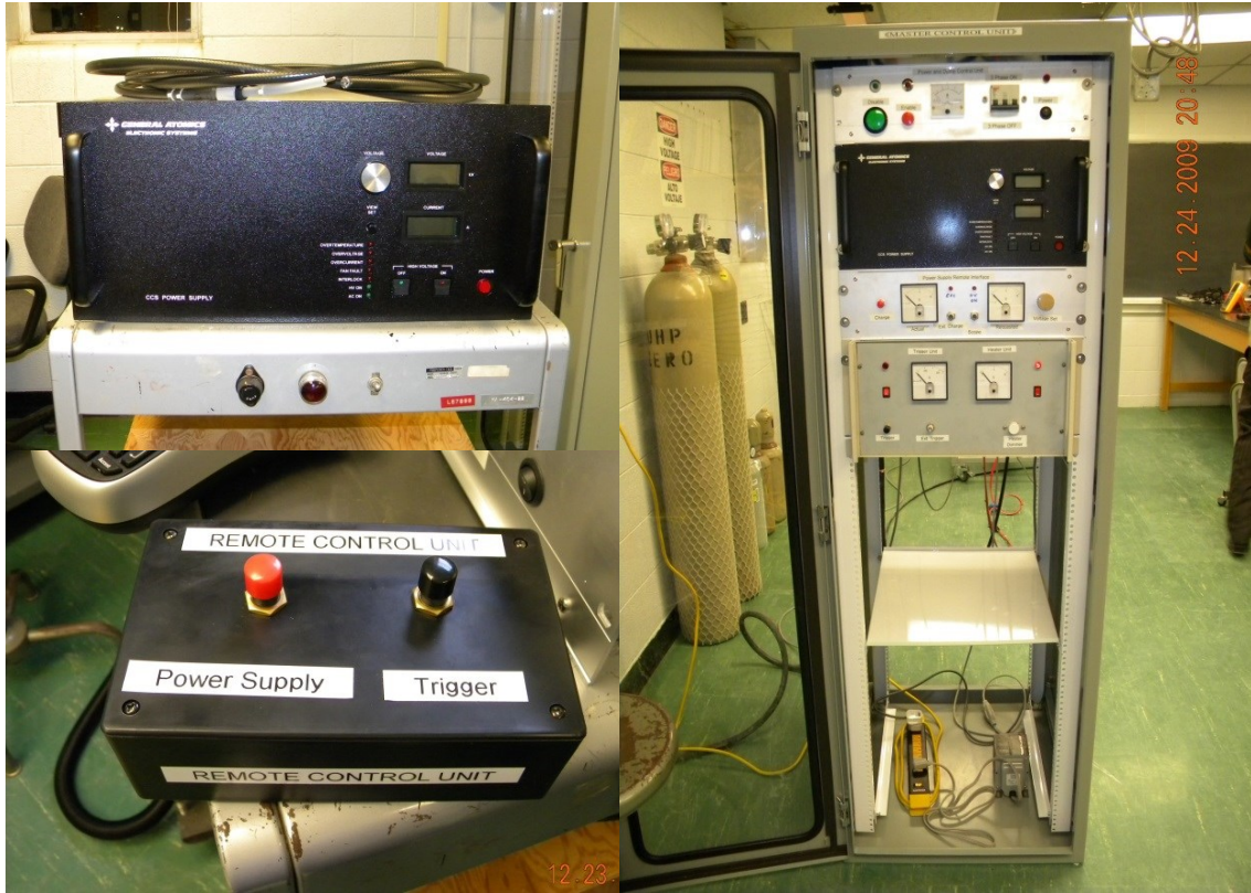
Figure 3-8. The power supply (left-top), its remote control (right-bottom) and the cabinet (right).
