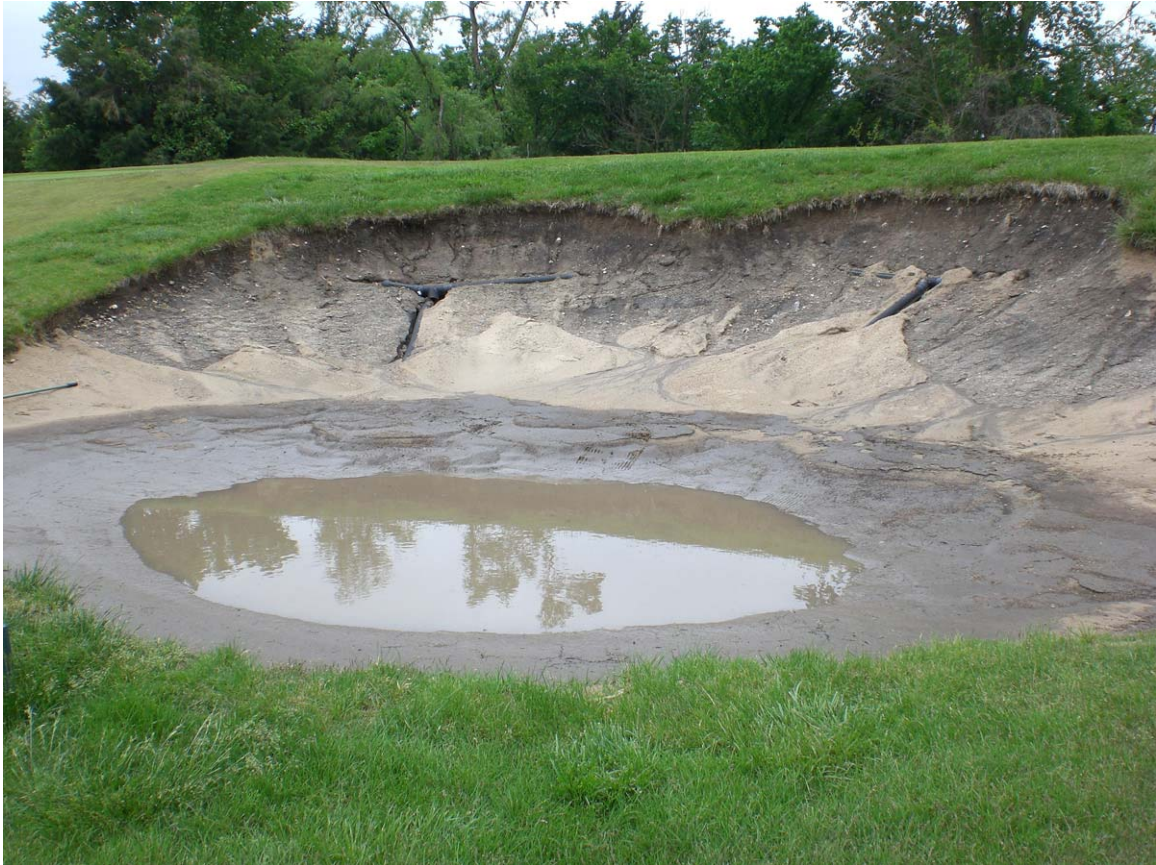
Figure 2.60 – Bunker Erosion and Standing Water, Colbert Hills Golf Course, Manhattan, Kansas (Author)
