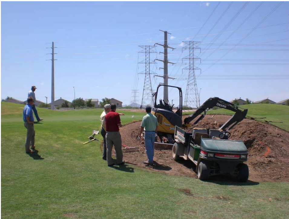
Figure 2.34 – Architect Supervision of Bunker Construction, Hole 2 Coldwater Golf Course, Avondale, Arizona (Author)
