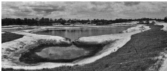
Figure 2.5 A lake with a smaller phytozone under construction (Libby et al., 2004, p.50)
