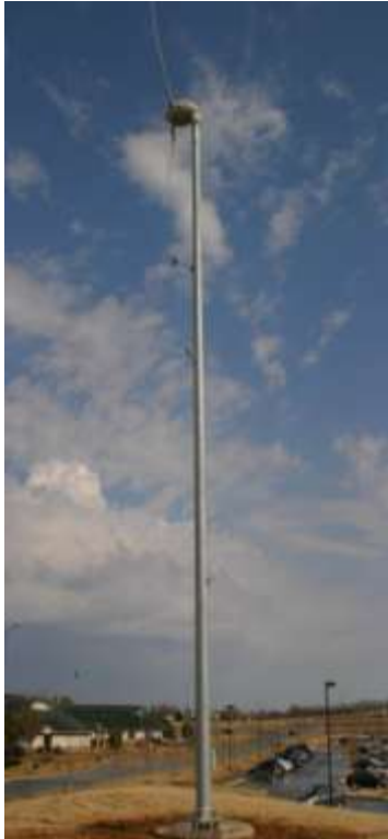
1.8 KW Wind Turbine
